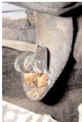
Photo #4 - Plugged Drain Tube!
