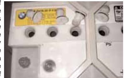
Photo #4 - Cell Caps Removed For Electrolyte Check
